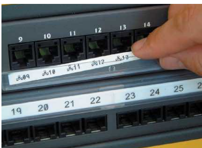
Punch block & patch panel labels
